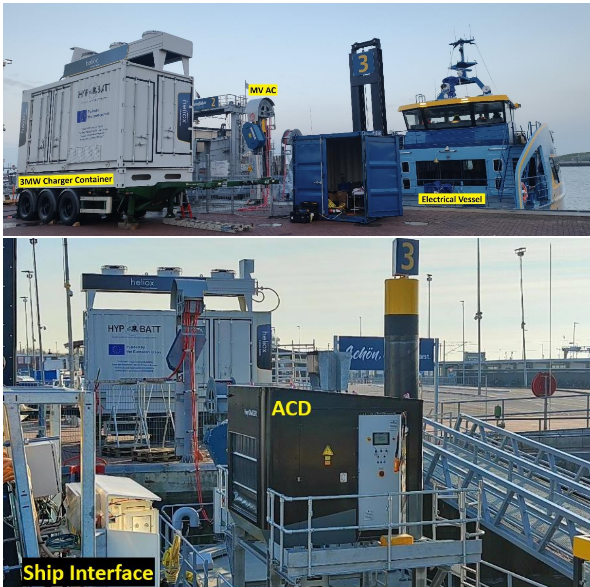
Figure 3 overview of the mainland system EVSE 1 test installation and equipment placement at Frisia site.
