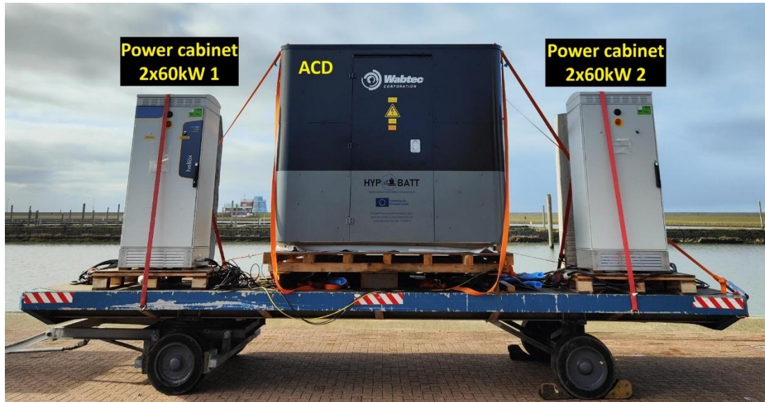
Figure 4 Overview of the island system (EVSE 2) test installation.
