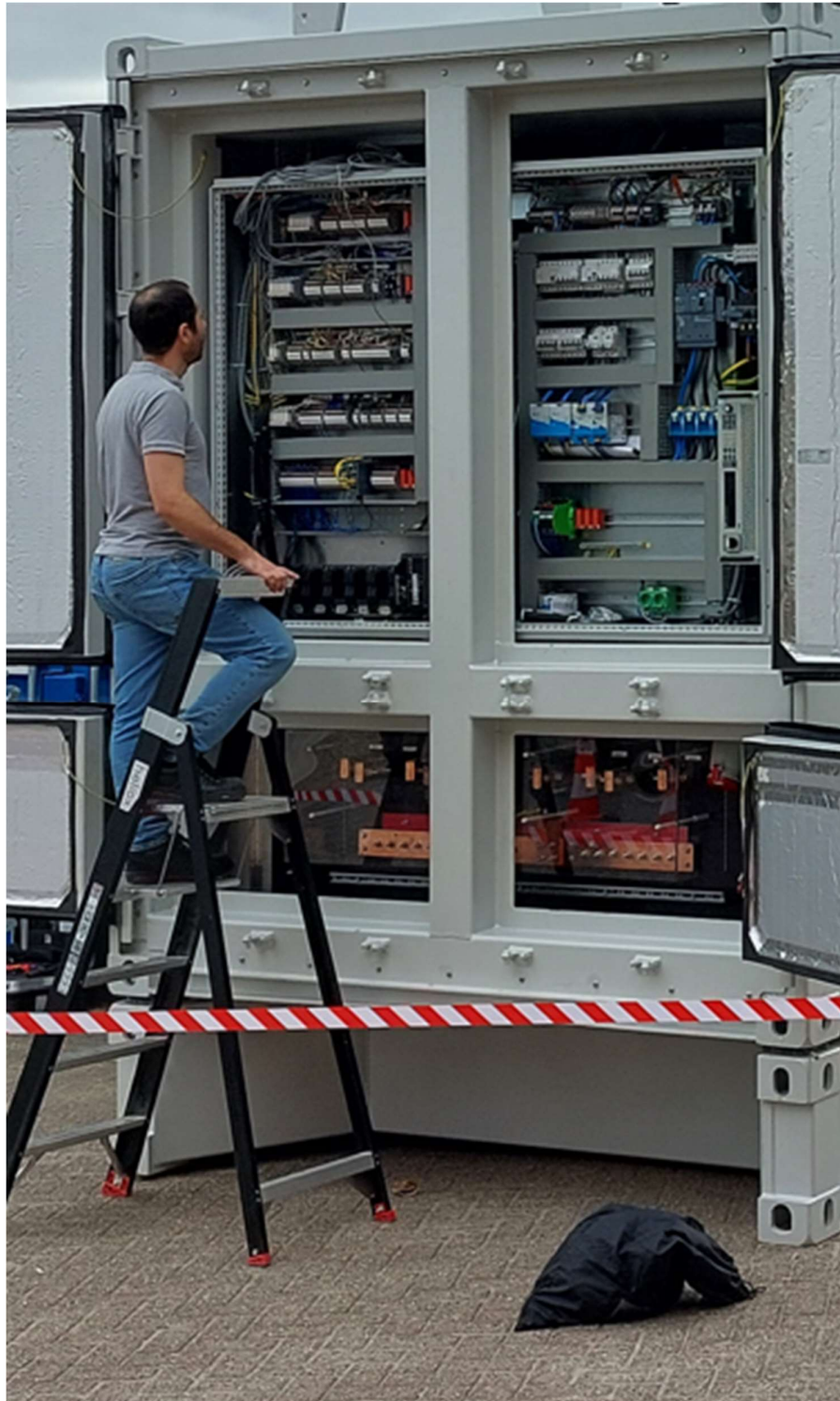
Figure 8 LV DC and control side during installation check and testing start-up
