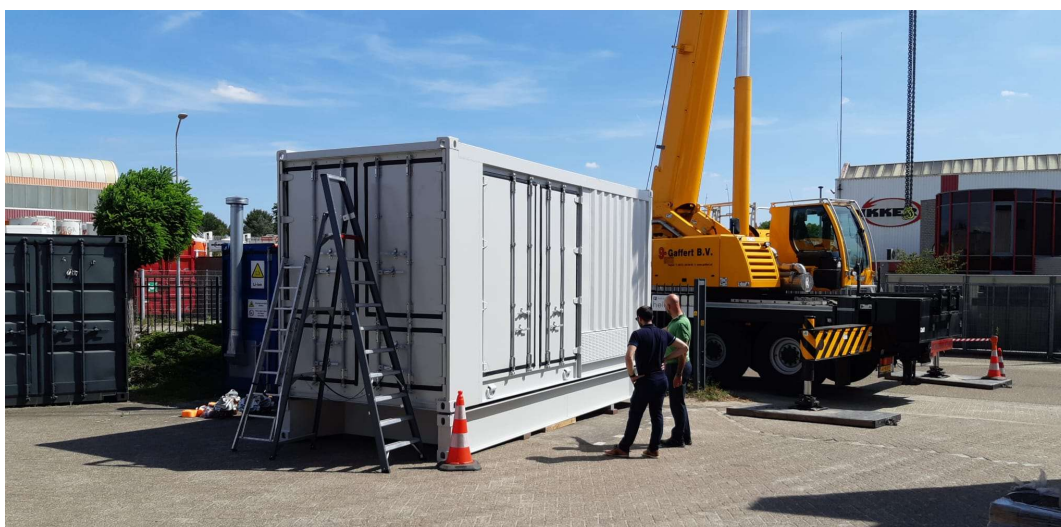
Figure 2 placement of the multi-MW charger on the baseframe
