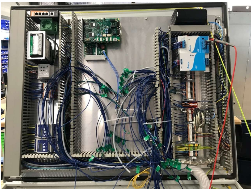
Figure 11 internal control section of the DC outlet dispenser (missing the central controllers still)
