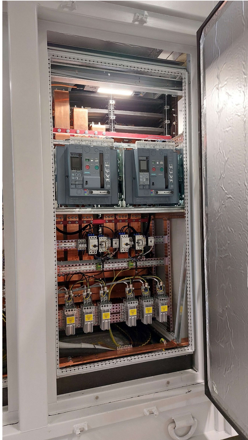
Figure 9 LV AC air-circuit breakers and pre-charging compartment
