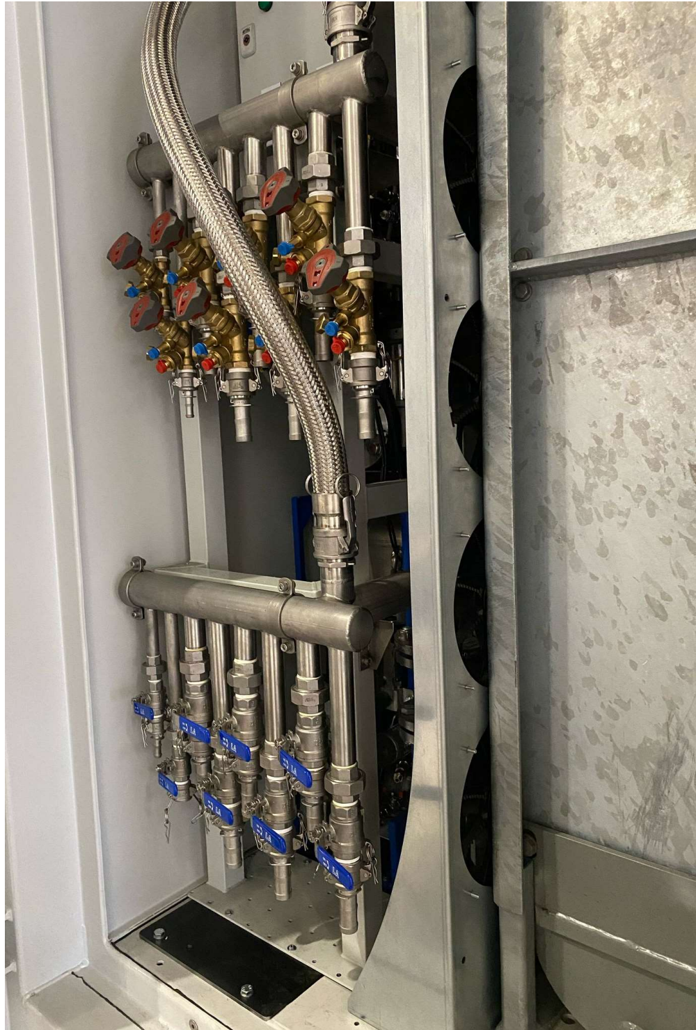
Figure 6 cooling station with left: manifold supply (top) and return (bottom), behind that the pumping station, right: heat exchanger with fans.
