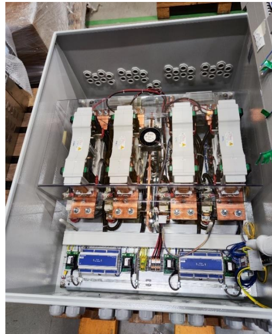
(b) picture of the implemented power section
