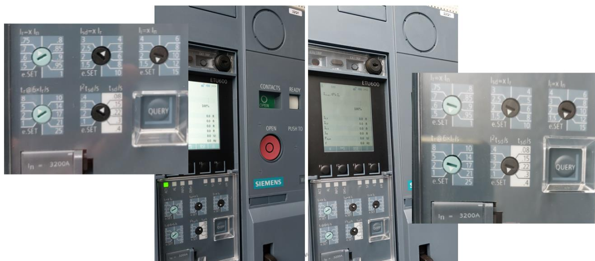
Figure 8 AC 3200A ACB protection settings (acc to fig 7 in short-circuit calculation settings 24PPR1234)
