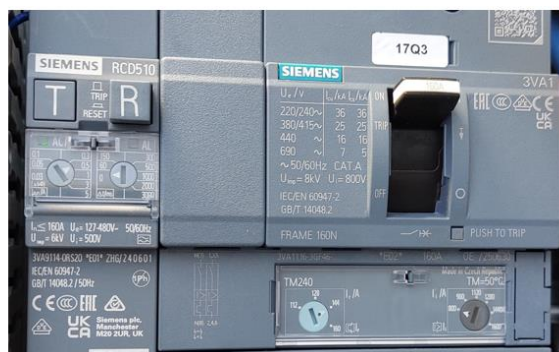
Figure 9 AC 160A ACB protection settings (acc to fig 9 in short-circuit calculation settings 24PPR1234)
